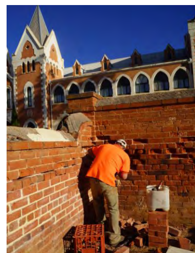
Image above; Shane working on the wall. See left of the image for a finished piece of restored brickwork.
