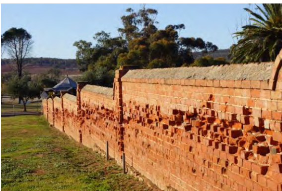
Image above; the full extent of the restoration needed.
